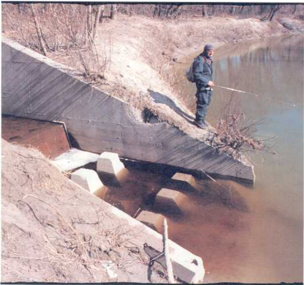
Rouge River — polluted storm sewer run-off
